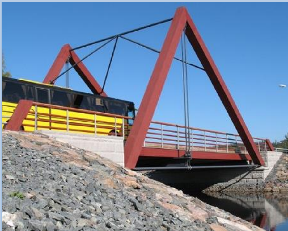
Figure 21. Wooden bridge in Virserum (Sweden) designed and built based on the new bridge construction standards in Sweden
