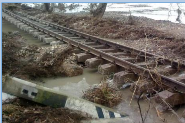
Figure 11. Damaged railway line due to flooding (2014)
