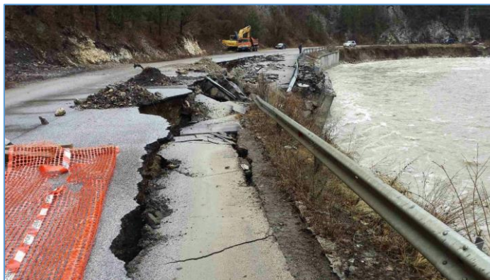
Figure 10. Damaged embankment and road due to a river flood (2015)
